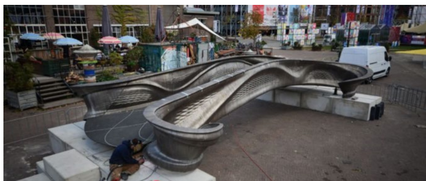
Fig. 1. A stainless-steel bridge construction, made with the use of an automated 3D print technology
